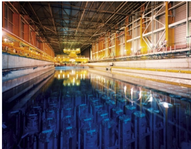
AGR spent fuel storage pond at Sellafield
