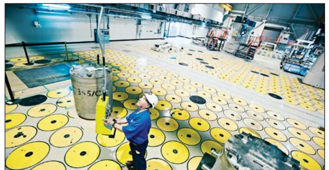
Inside the Vitrified High Level Waste Store
