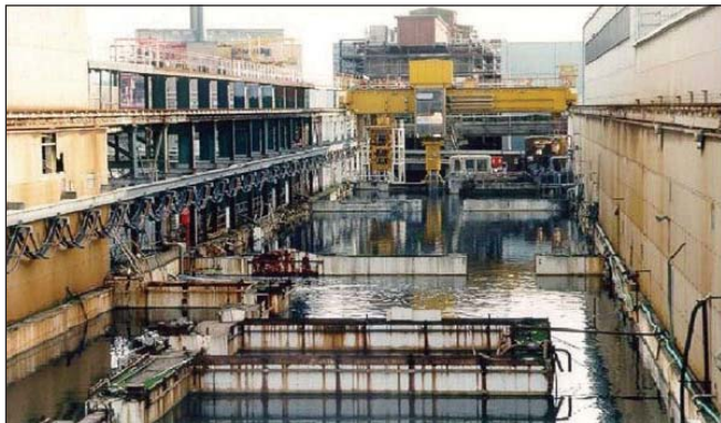
Old nuclear fuel storage pond
