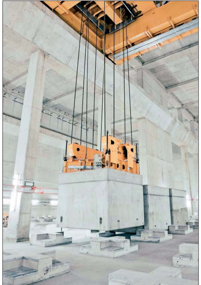
Inside the ILW Store at Trawsfynydd
