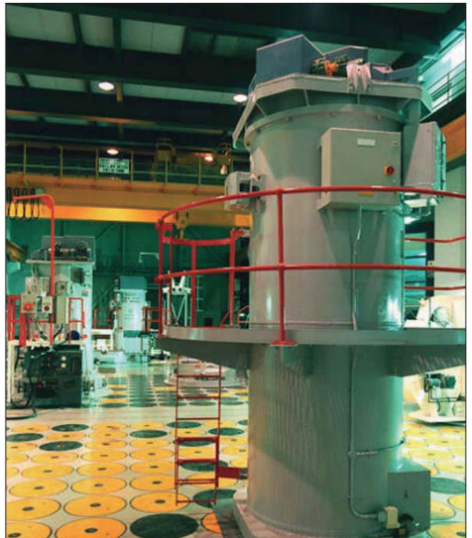
Store for packaged HLW canisters
